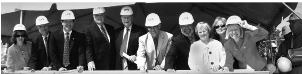
Signing their names to the final piece of steel before it is hoisted to the top of the building are (from left): Stephannie Beemer, chief of staff to state Sen. Andy Dinniman; Peter Kaplan, vice president for PNC MultiFamily Capital; Congressman Jim Gerlach; State Rep. Tim Hennessey; Albert Eastburn, chair, Brandywine Health & Housing Center; Harry Walker, Coatesville city manager; County Commissioner Pat O'Donnell; Anne Hearn, chair, Brandywine Health Foundation; Betty Randzin, district director for state Sen. John C. Rafferty Jr.; and Frances Sheehan, president and CEO, Brandywine Health Foundation.
